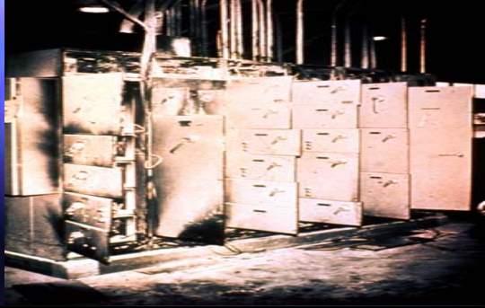
Electrical Switchgear - Arcing
