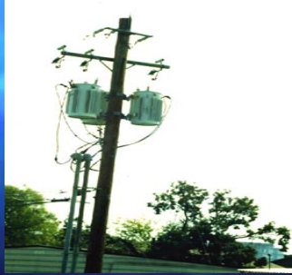
Pole Mounted Transformers
